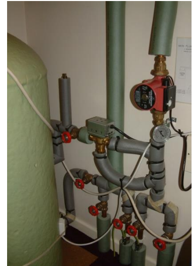
Original heating pipework and controls
