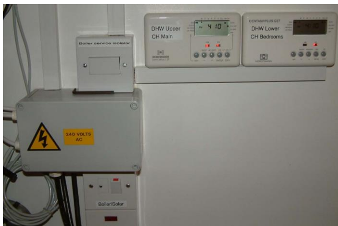
Twin programmers and electrical control installation
