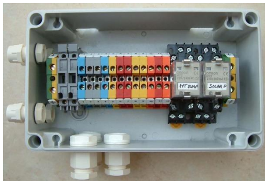
Main wiring terminal and relay box for combined heating and solar wiring
