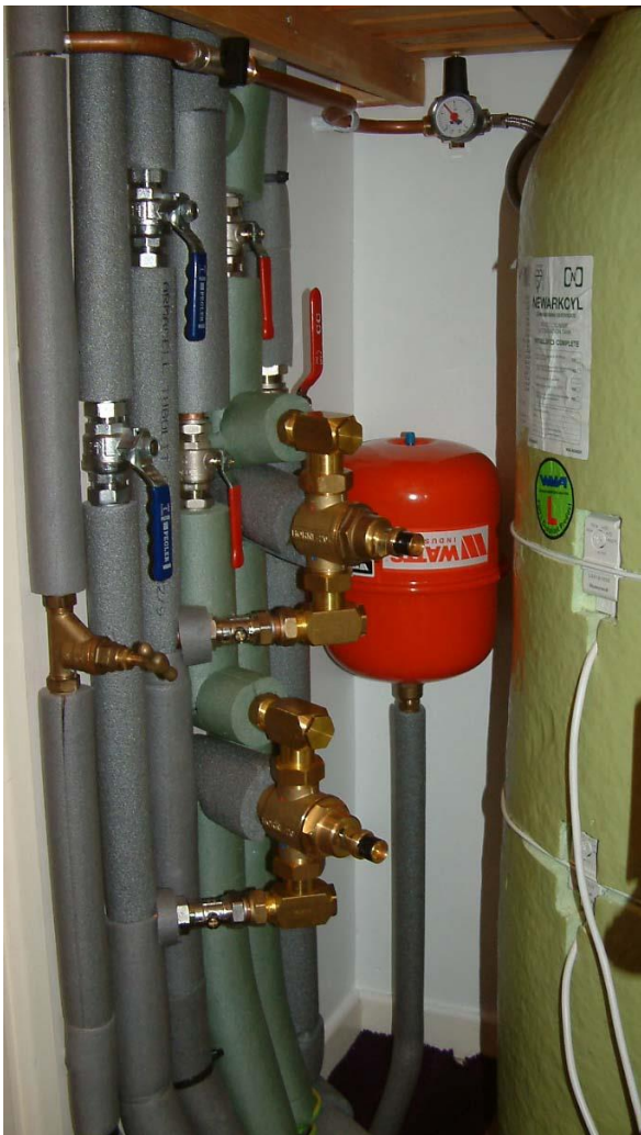
New valve gear and TMVs – part of solar filling-loop and Pressure Regulating Valve at top
