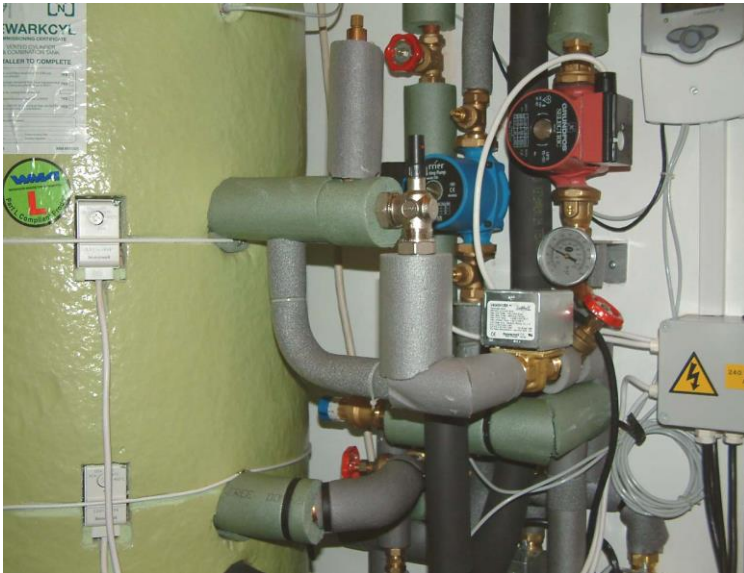
ADPBV detail on boiler coil – main system ADPBV in background (blue cap)
