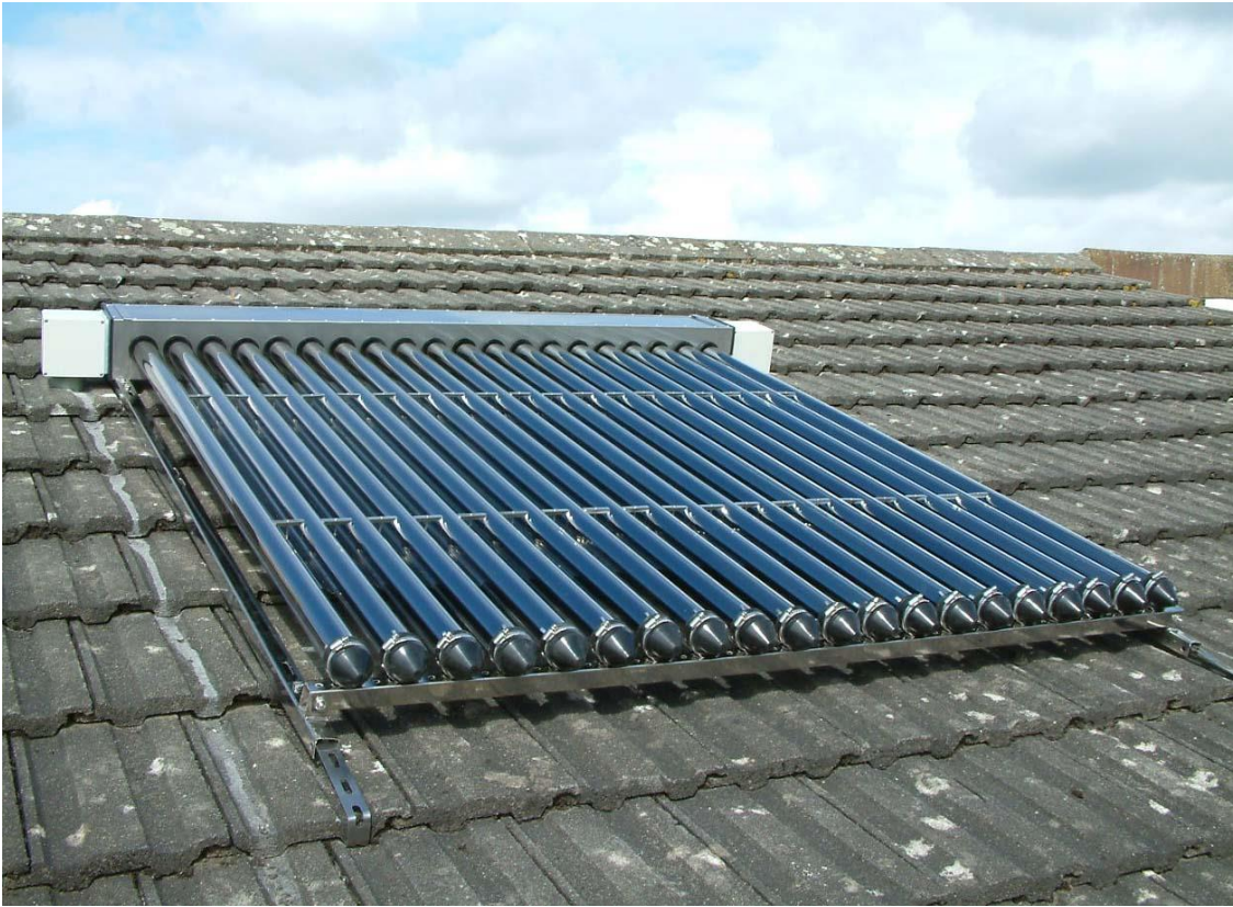
The installed solar panel complete
