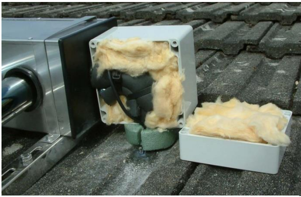
Right-hand end cap box internal view
