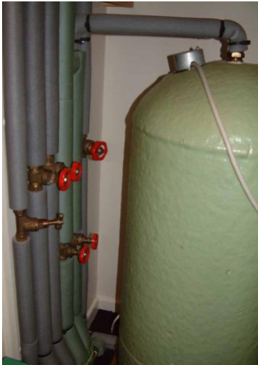
Original installation water feed pipework
